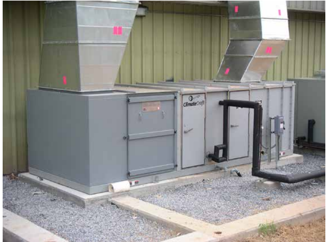
Anniston, AL – Custom Air Handling Unit with Single Attack Chemical Adsorbers
